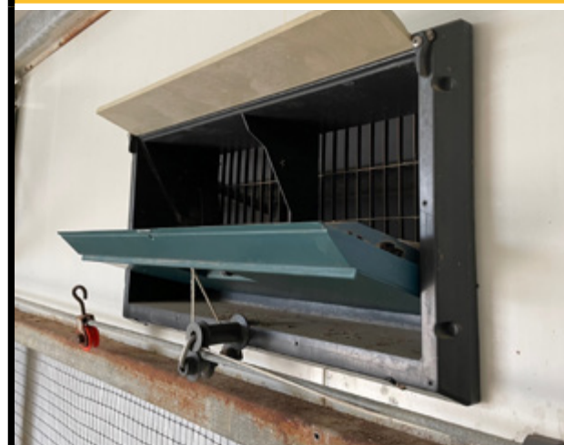
Figure 100 Example of a good-quality air inlet.
