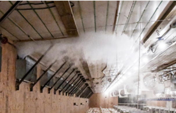
Figure 105 Using a smoke test to determine if air flow and operating pressure are correct.
